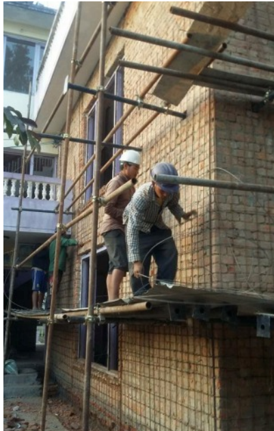
The laborers are working hard on retrofitting our House to make it withstand future earthquakes. It is a lengthy and messy process!
